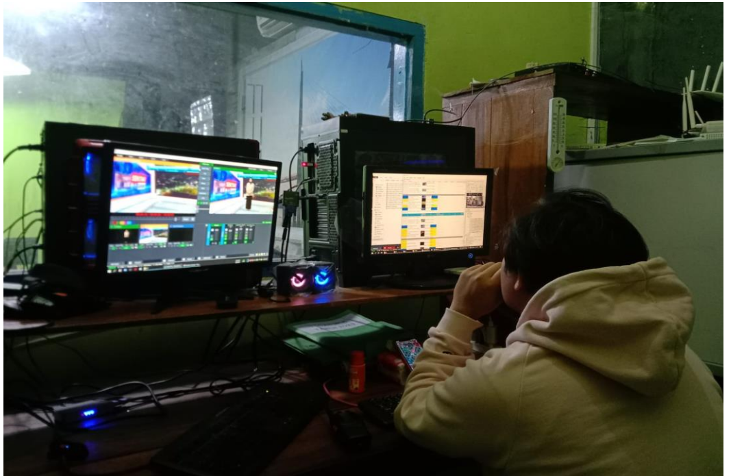
Gambar 2 : Master control room (MCR)
